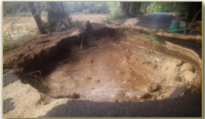
A sink hole on the road.
