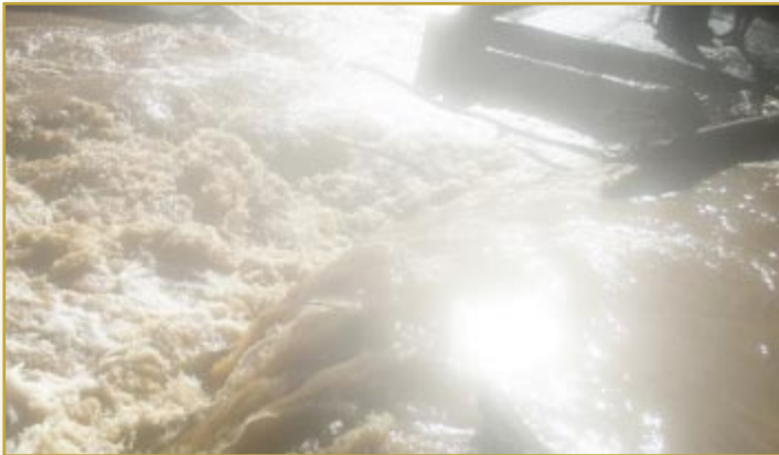
A large central section of the bridge across the Tweed River has been washed away.
