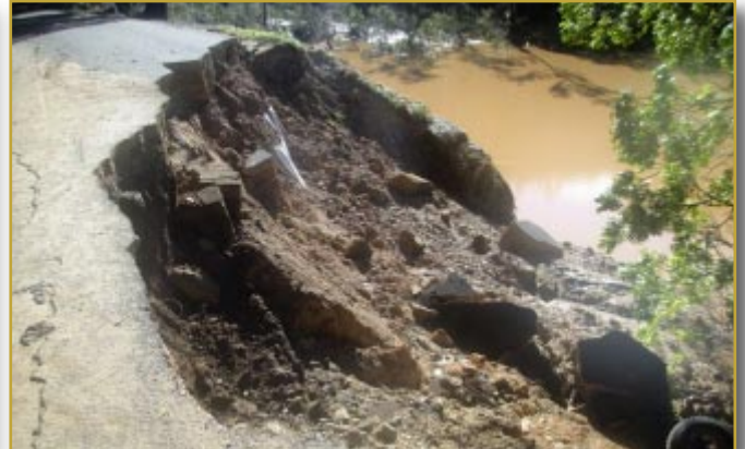
Part of the only road out of here has eroded and fallen into the river.
