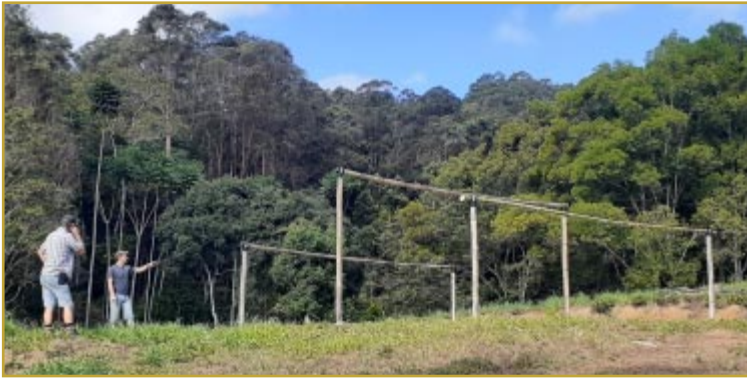
Above: The beginnings of a structure on the land. Below: Sebastian and Jeremy at work...
