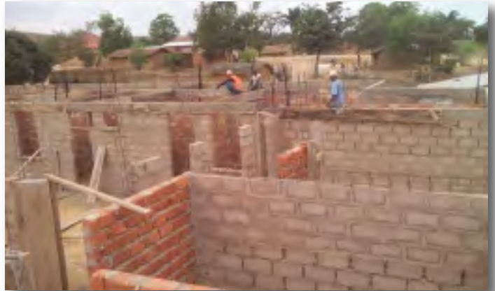
Work in progress on the Kwilu Ngongo Mother-Child hospital that Melina is fundraising for.
