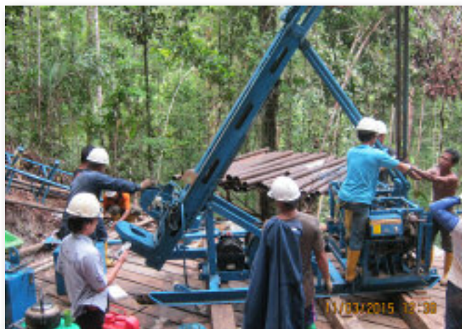
The drilling crew setting up one of the company owned and operated drill rigs.
