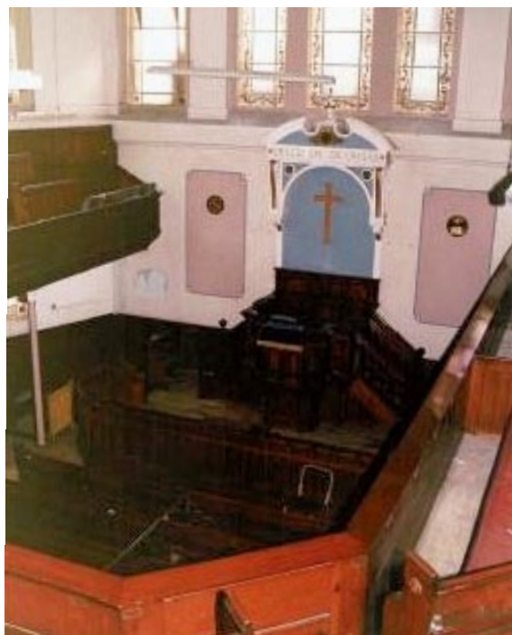
Interior of the Amadeus Centre at the time of purchase. It had been a church.
