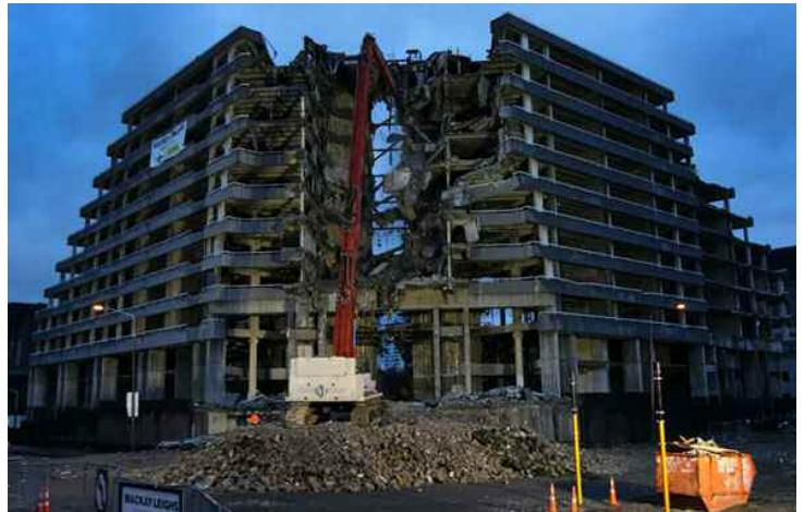
The Crown Plaza Hotel where Ibu Rahayu stayed during World Congress next to the Convention Center is now under demolition along with the Convention Center.
